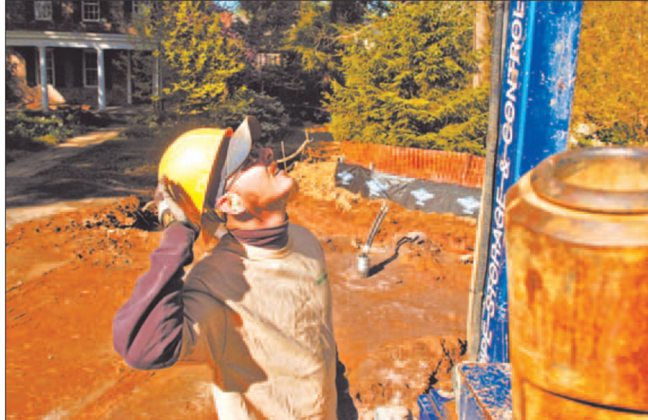
MATT STANLEY / STAFF PHOTOGRAPHER Matt D. Snedcker of Jackson Geothermal drills a 540-foot well to be used as part of a heating and cooling system at a 170-year-old Newtown building being "greened" before becoming the headquarters for the Creative Strategy Group, Inc.
